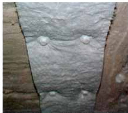
CLOSE SHRINKAGE GAPS
